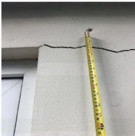
Crack above rear door.
