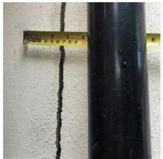
Crack on rear wall.
